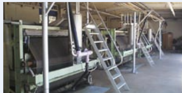
These Belt Presses operate 24 hours per day
