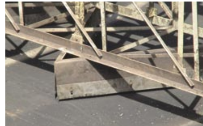
Rubber components wear frequently
