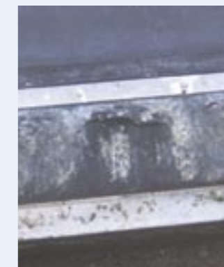
A close up of the damaged hinge
